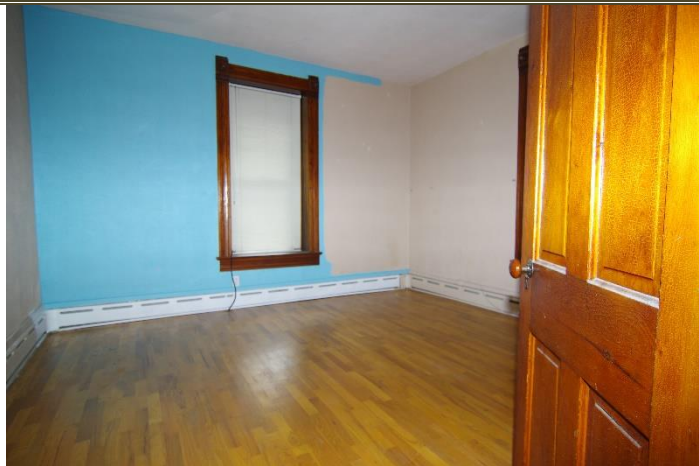
Dining room showing refinished wood floor, wood window trim and doors, and the start of a repaint.
